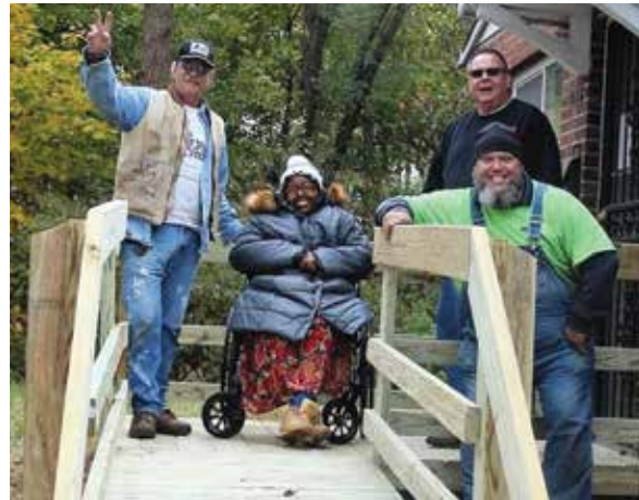
One of four ramps completed by SAWs in Lake County's first build season.
