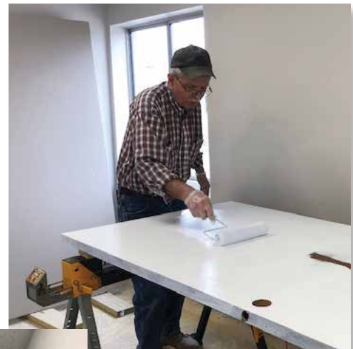
Jim Hamilton, Area Coordinator and Project Manager for the renovation, rolls up his sleeves.
